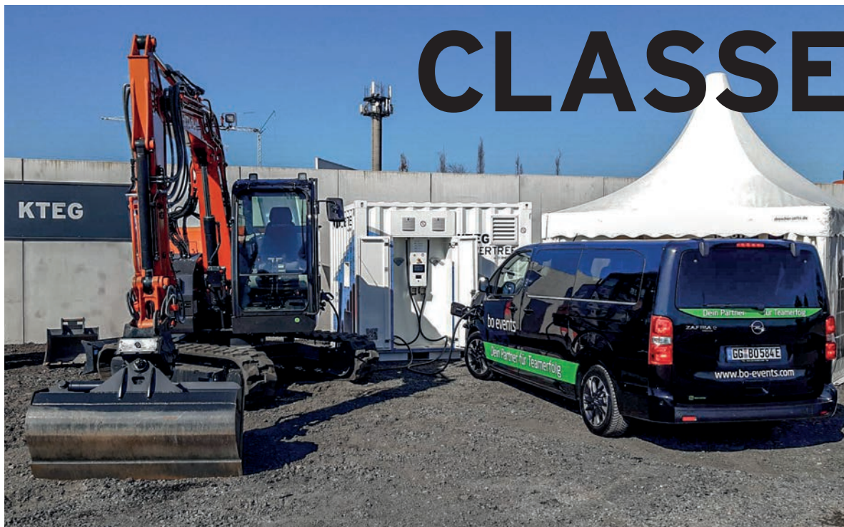
Even electric vehicles can recharge at the Powertree.
